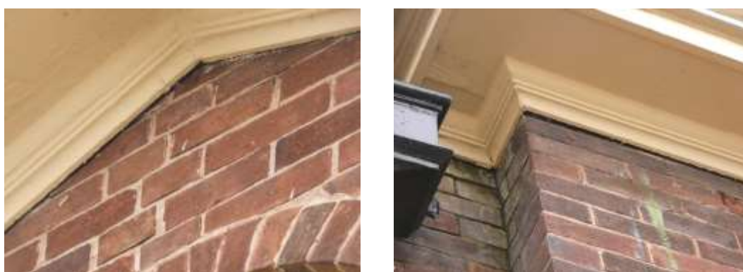
Figs. 11 & 12 Auction House – examples of soffit gaps
