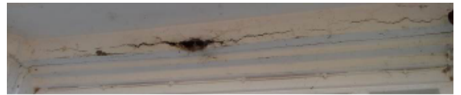
R8 – Cracking above front door
