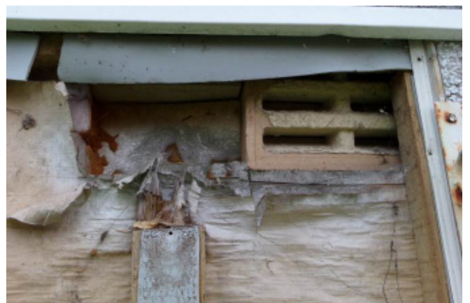
R12 – Perished membrane at un-sleeved vent
