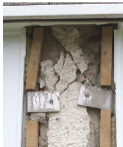
R6 – Original render cracked & spalled, damage to PRC beneath
