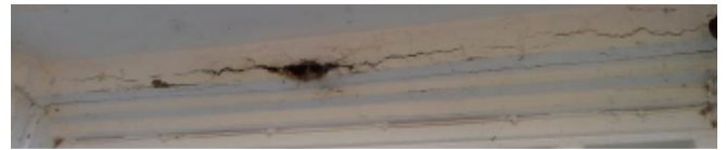
R8 – Cracking above front door
