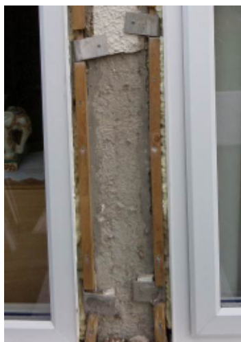
R5 – No insulation between windows original render spalled off
