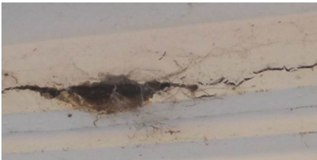
R9 – Cracking detail
