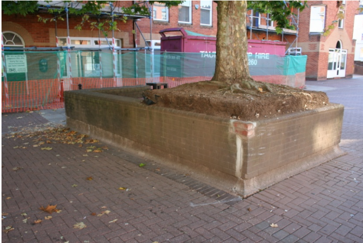
Strangled rootbound trees breaking their planter & possibly unstable
