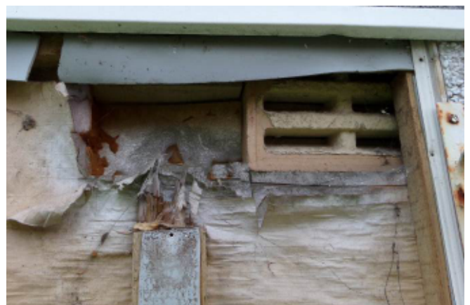
R12 – Perished membrane at un-sleeved vent
