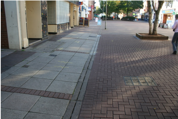
Uncoordinated paving and materials
