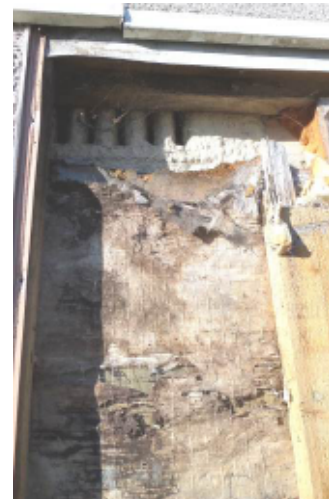
R10 – Perished membrane at un-sleeved vent
