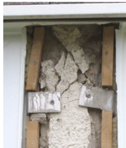
R6 – Original render cracked & spalled, damage to PRC beneath
