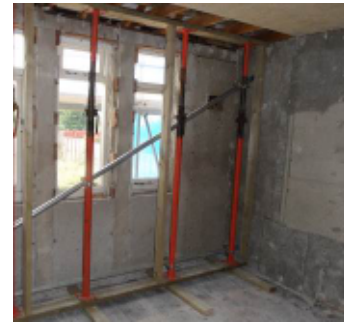
R16 – First floor rear external wall (left) & party wall with adjoining property (right) after inner lining removed
